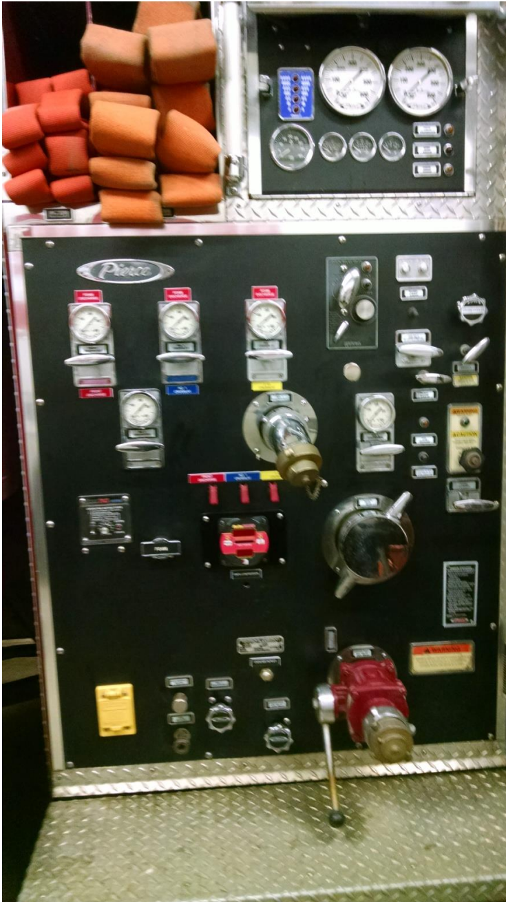
Engineering Control Panel
