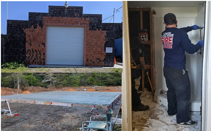
Clockwise from top: 1) Exterior of Station 810 with raised roof 2) Masked firefighters worked with board members to demo old 810 bathroom 3) New slab poured at Station 812 next to the airport.
